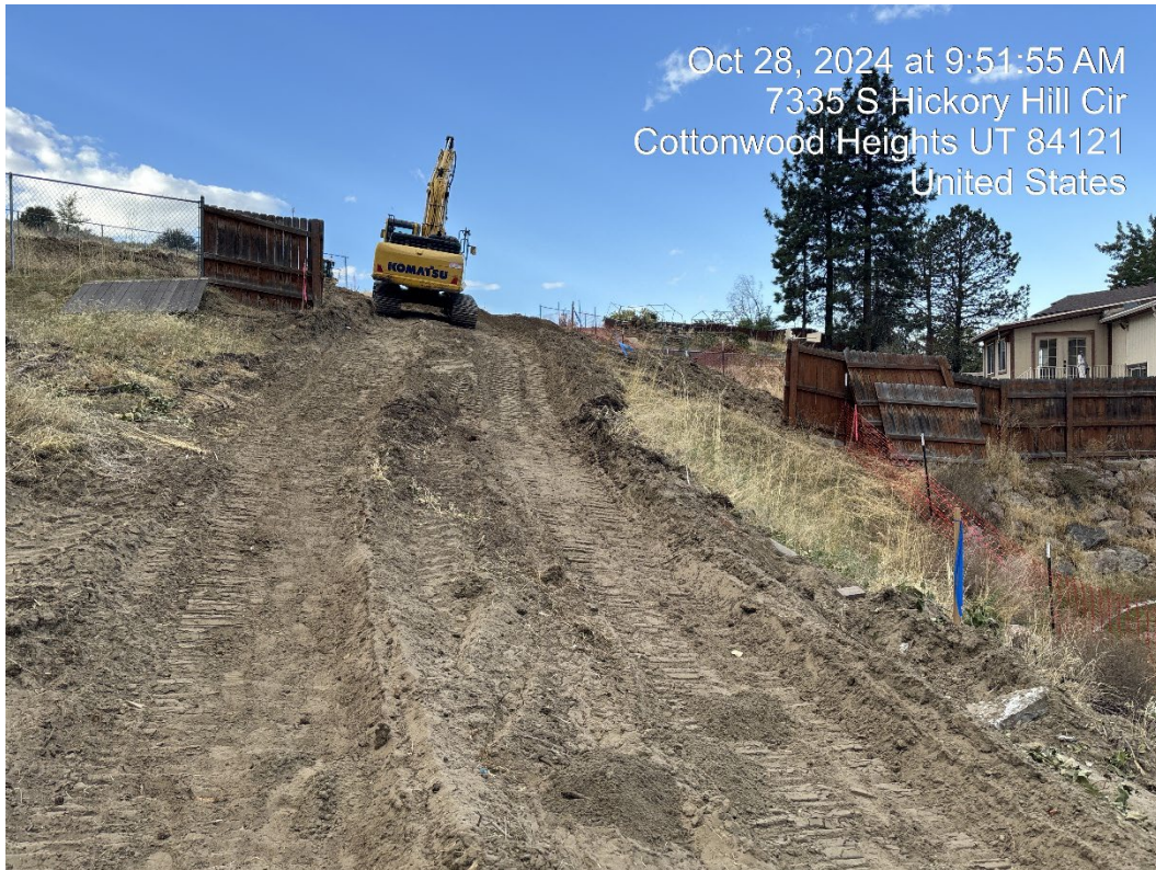
October 28: The contractor is preparing access to the Little Cottonwood Conduit through yards.
