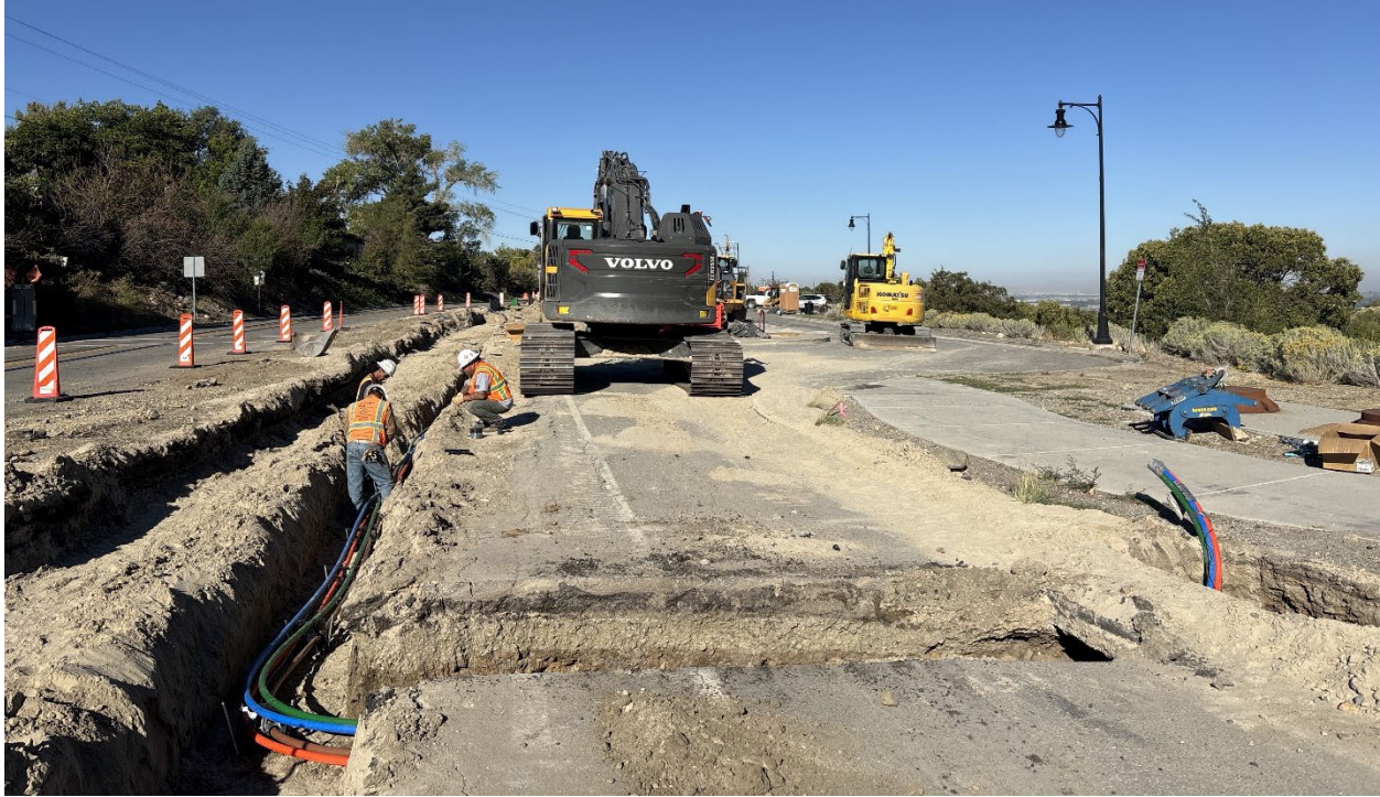
October 4: Utility conduits are installed above the pipe (and to a pull vault).
