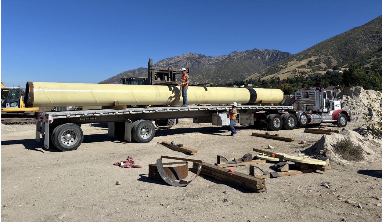
October 1: Pipe is loaded at the LCWTP to be taken to Fort Union for installation.
