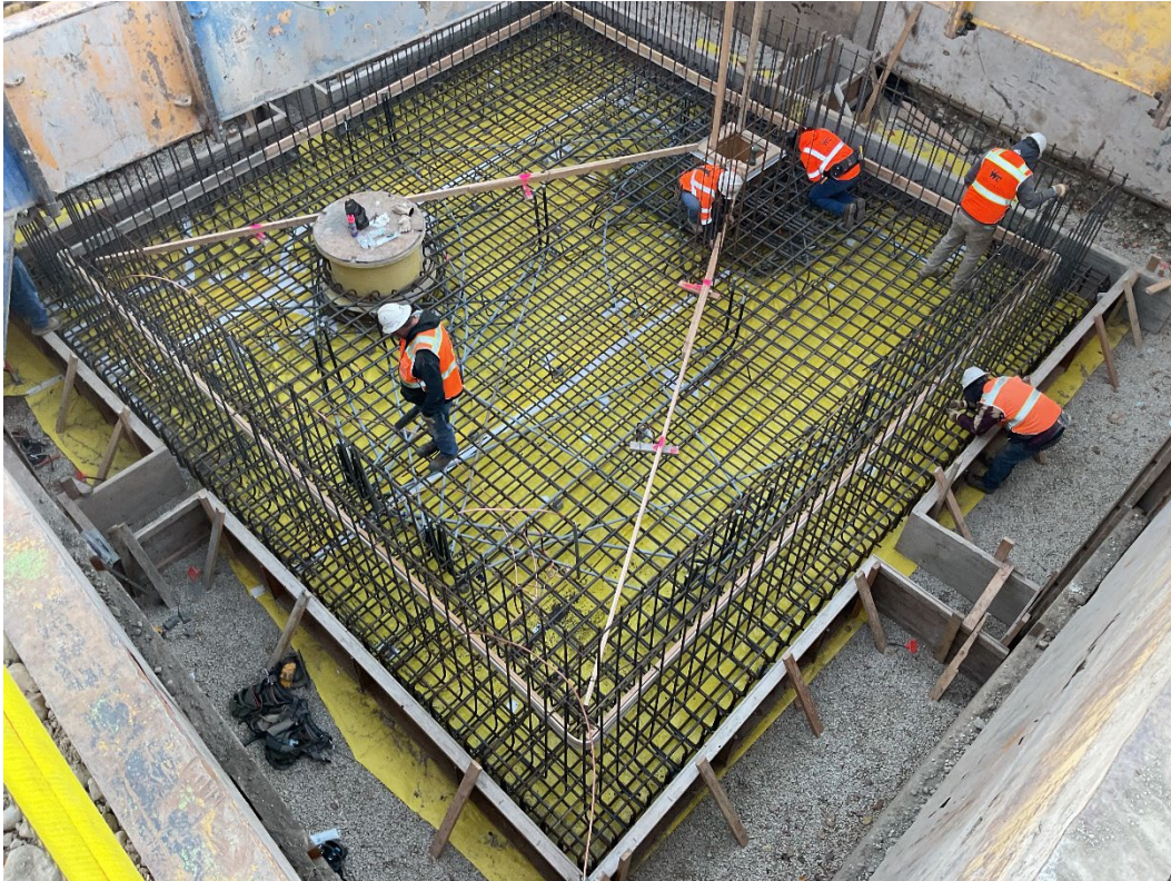
December 20: Floor rebar was tied and inspected in preparation for concrete at the CC-1 Vault.
