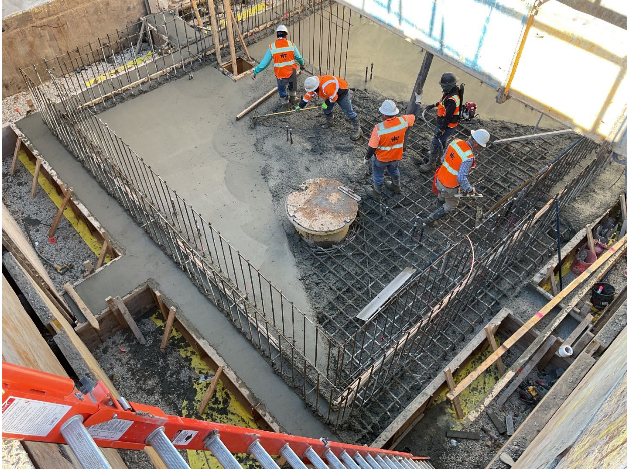
October 28 and 30: Excavating and pipe installation for the CC-1 vault is underway.
