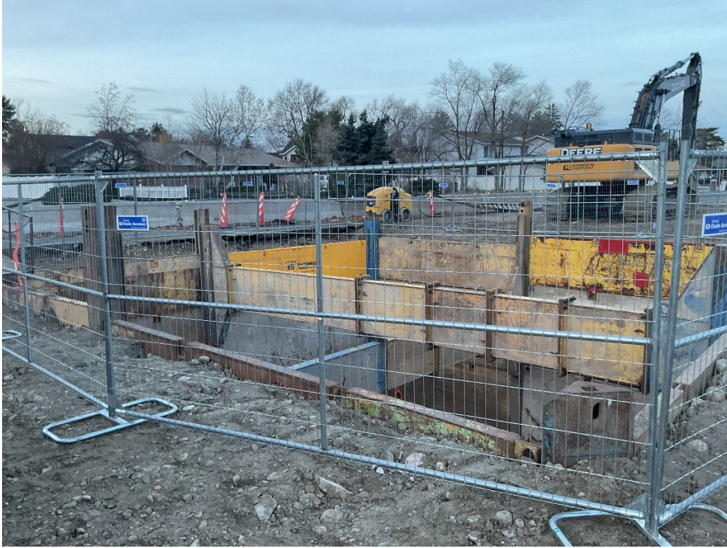
December 16: Framing and excavation for the CC-1 Vault at Fort Union and Nutree is underway.
