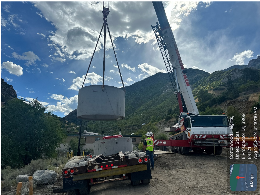
August 23: Manhole sections were received and placed for a manway access on CC-1 near the BCWTP.
